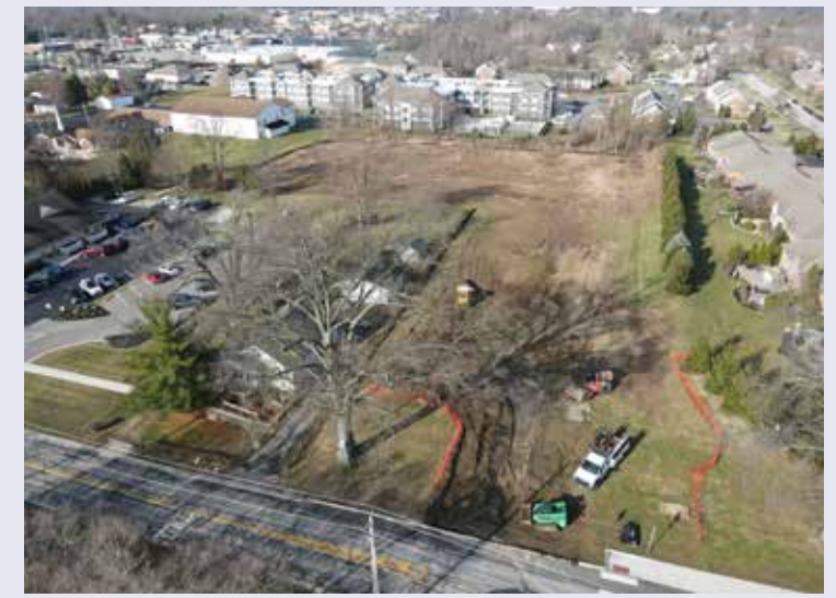
Nagel Road site development is underway on a property previously owned by Anderson Township.
